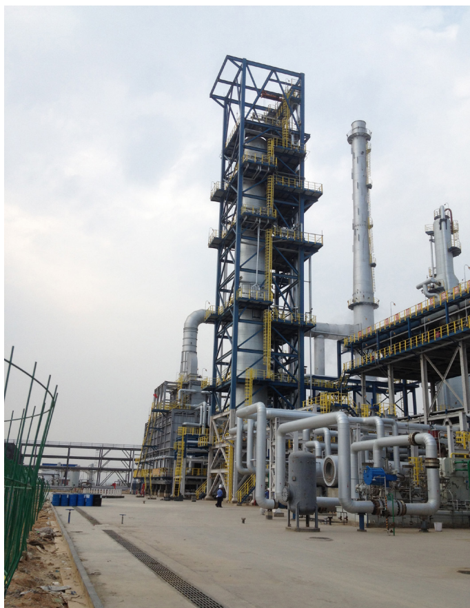
Figure 1. An IsoTherming reactor in commercial service.
